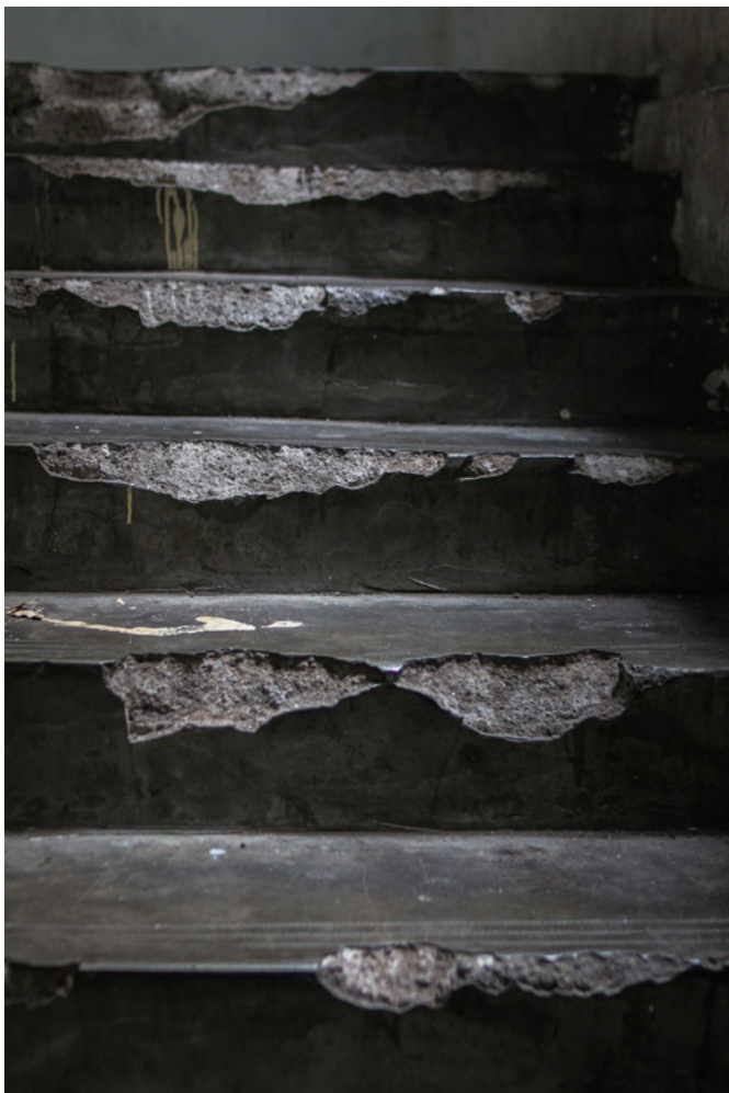
Figure 16 Hazardous stairwells at a PPR
