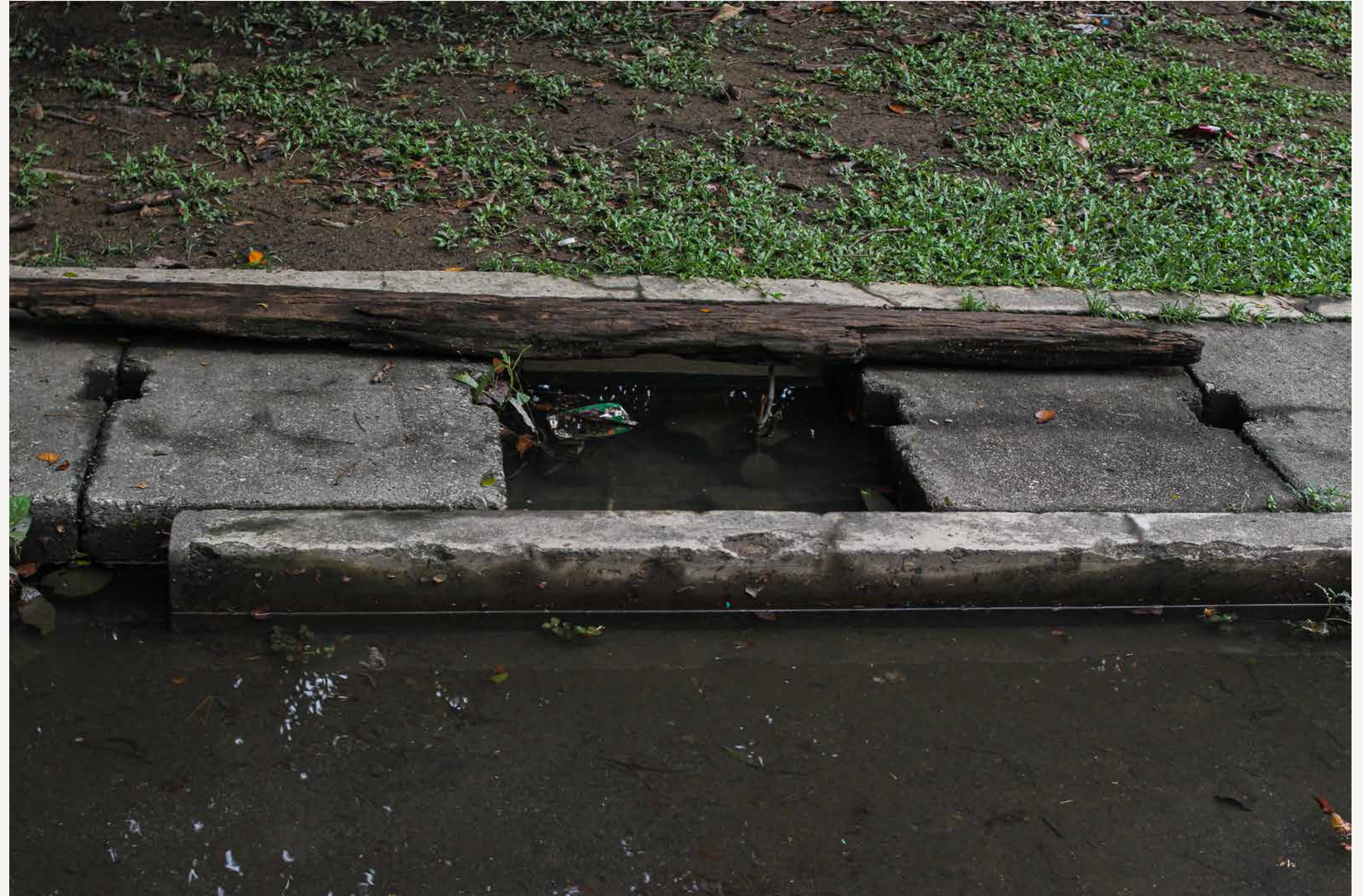
Clogged drain with stagnant water becomes breeding grounds for mosquitoes
